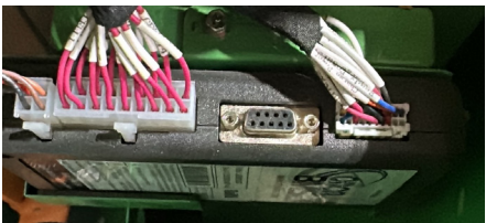
fig. 2A – BMS connection port.
